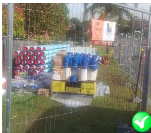
Figure 4 Pipes and fittings stored with protective caps
