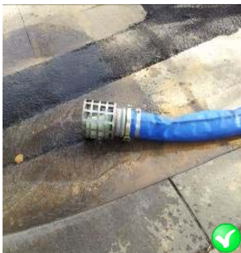
Figure 6 Discharged water & swab controlled
